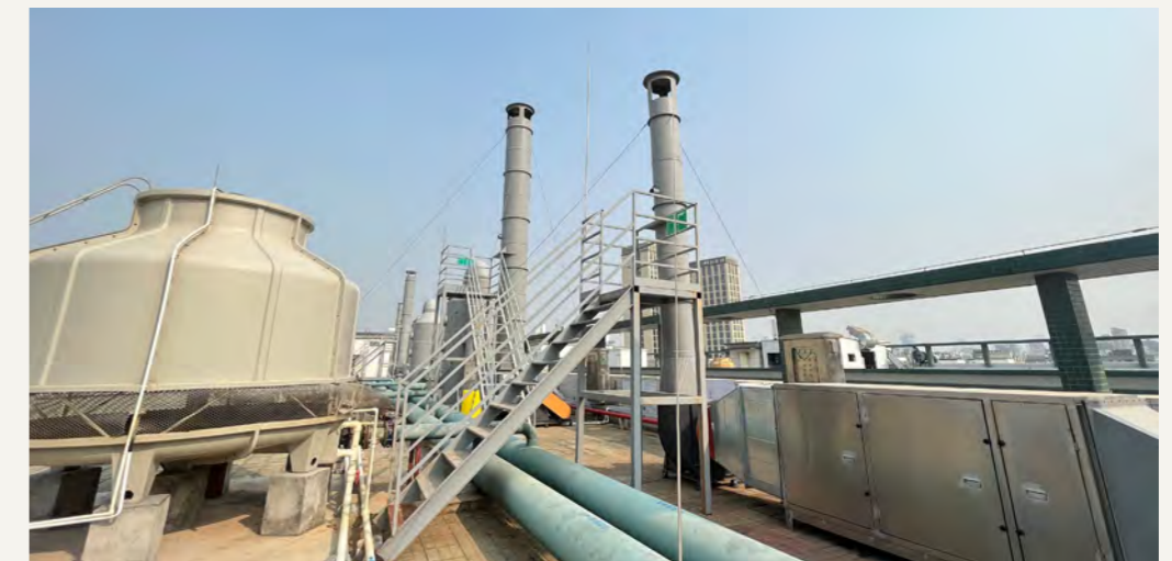
Exhaust gas treatment facilities
